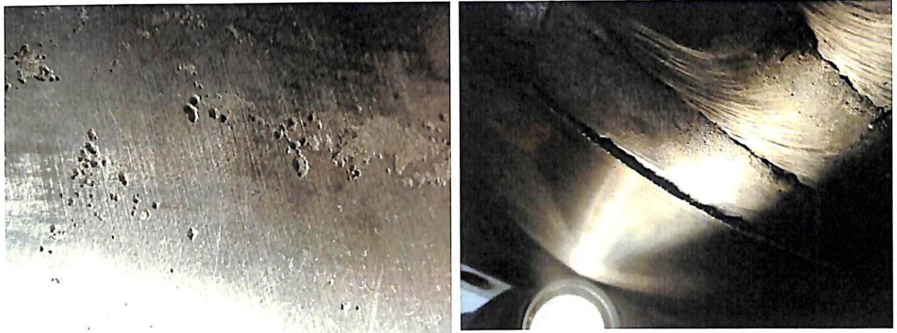
Figure 4.2: Plant Anomaly Snapshot: Off Gas Compressor 1 st Stage Suction Drum:
