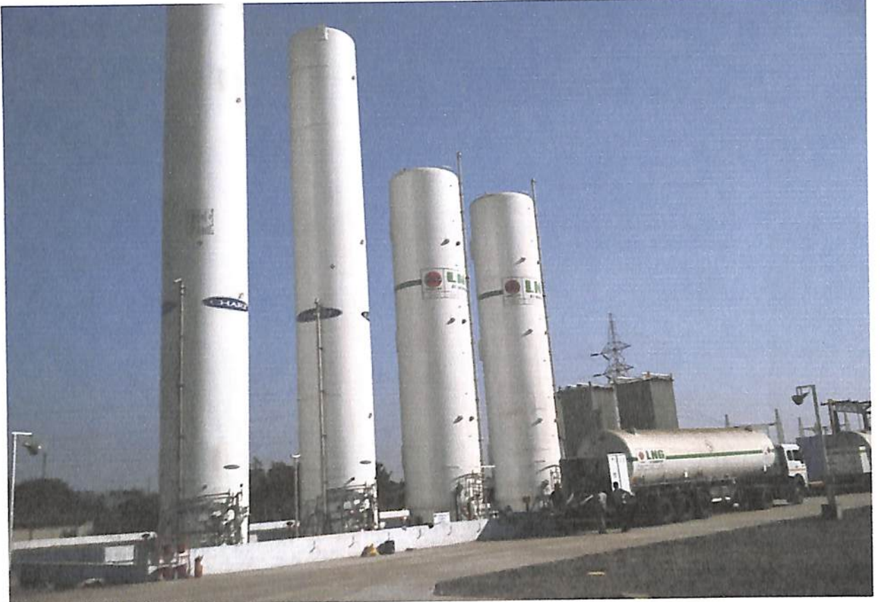
Fig5: LNG System at Hindustan National Glass, Sinnar (commissioned)
