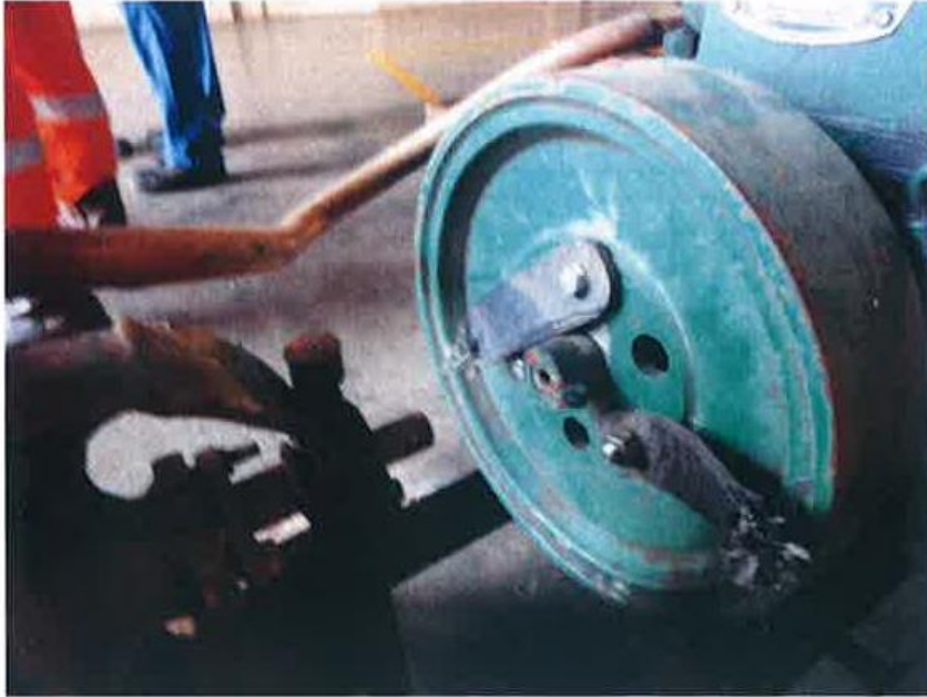
Figure 22: Broken coupling of Pump
