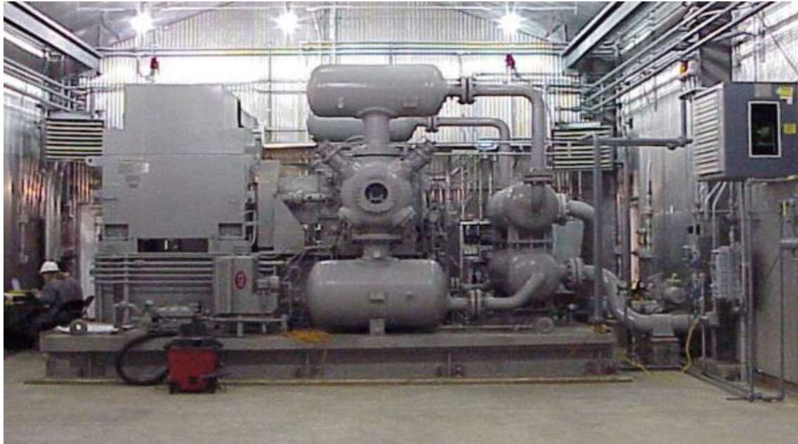
Figure A: Fuel Gas Compressor Unit
