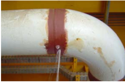
Figure 1.1b: Corrosion Failure at HAZ [1]
