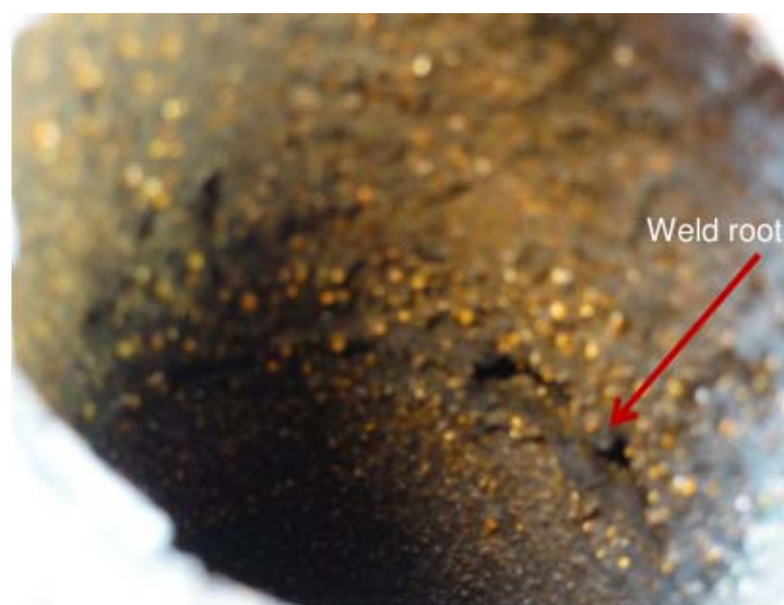
Figure 2.8: PWRC of Failed Pipeline
