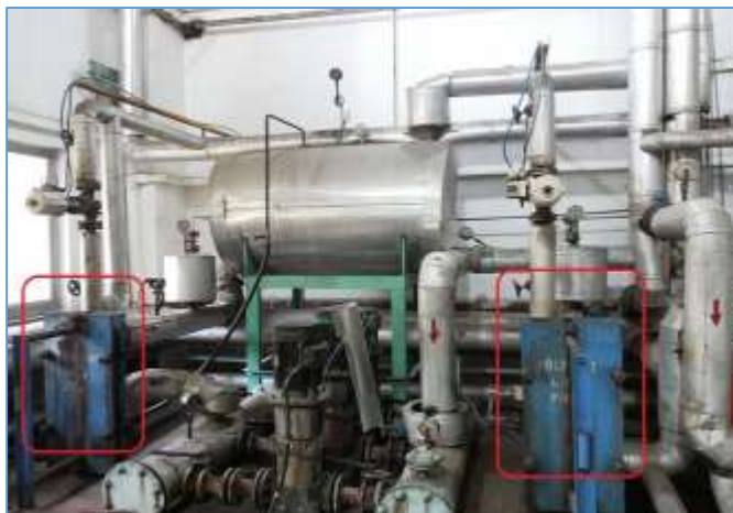
Fig 4.15 (e): Spg. Line and Polymer Line PHE
