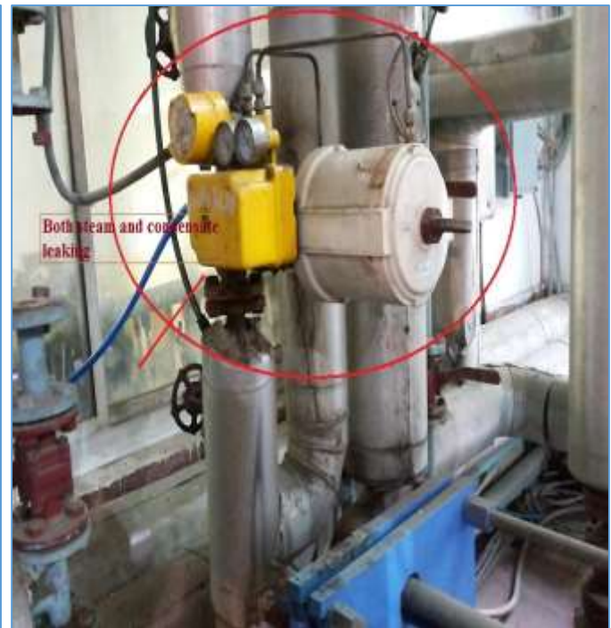
Fig 4.12: Steam Control valve of PHE 6
