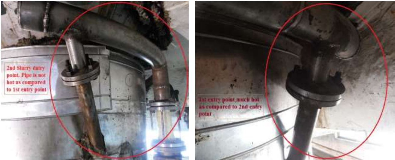
Figure 4.19: Slurry entry points to WFE
