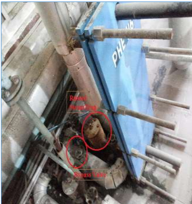
Fig 4.11: Steam trap and bypass valve of PHE 6
