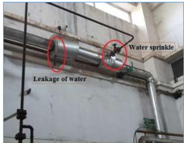
Fig 4.5(f): De-superheater water sprinkling
