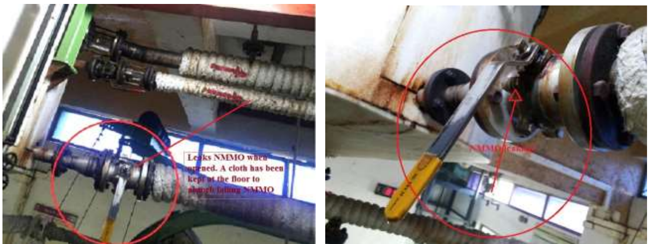
Figure 4.20: NMMO leakage from the hand operated valve
