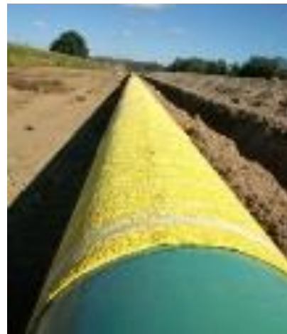
Fig 6.2.2 Rock Shield on a pipe
